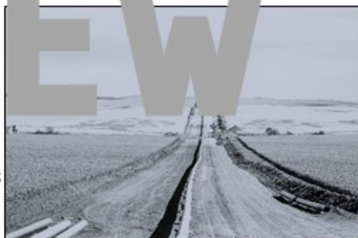
The Dakota Access Pipeline being installed between farms in New Salem, North Dakota
